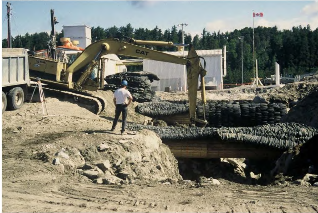
Figure 21: Blasting Under two high pressure gas pipelines, TransCanada Pipelines. Note 2x4 wood lagging around hotlines and blasting mats on top.
